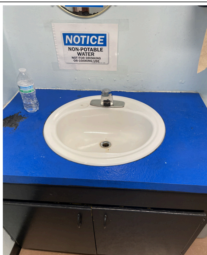
5/8/2024 - 527-4 - AG Building - Room F100c
